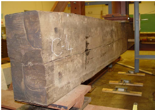
Figure 8: A horizontal shear crack (1).
