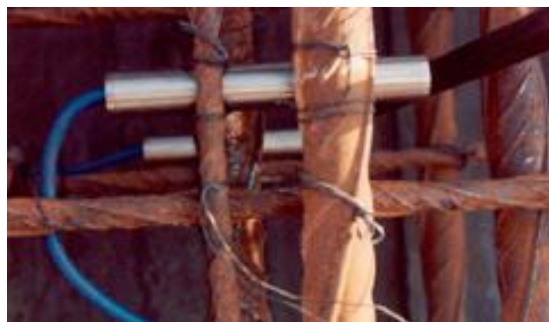
Figure 15- Structural health monitoring using Bragg grating [23].
